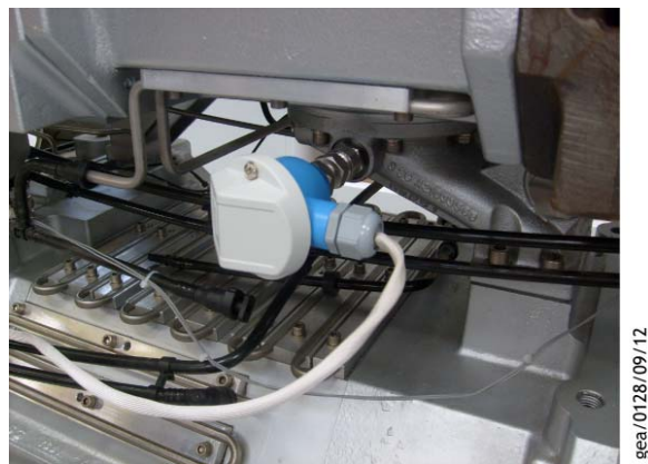
Figure 88 - Installation of the temperature transmitter to the spool between the pump and booster
